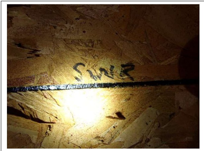
SECONDARY WATER BARRIER – A polymer adhesive (peel & stick) SWR Barrier was installed on the entire roof deck in 2018
