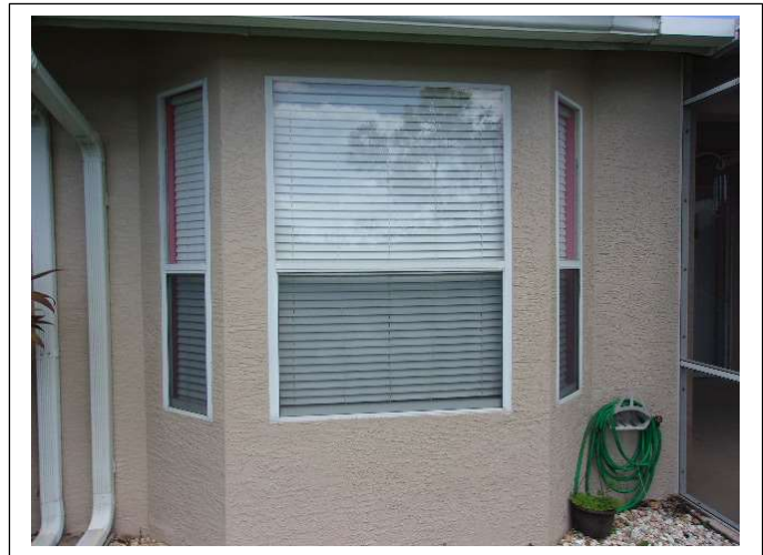
OPENING PROTECTION – Although some unit owners have installed wind-borne debris protection devices, others have not, leaving some openings (entry doors, window units and/or sliding doors) unprotected
